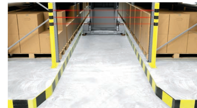
Stationary personal protective equipment with light barriers in selected rack aisles
